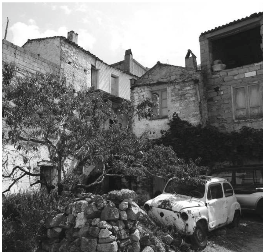
Fig. 1 The number of condemned building is progressively increasing ( source photo by the Authors)
